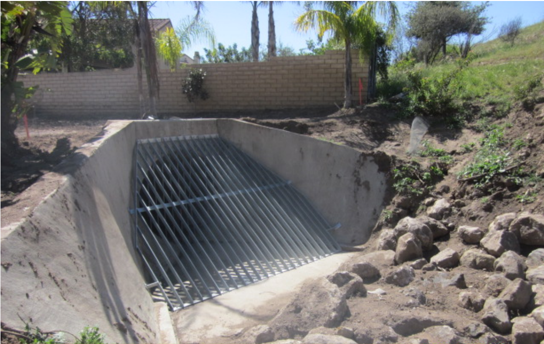
(Trash Rack_Large) (Trash Rack_Large)
