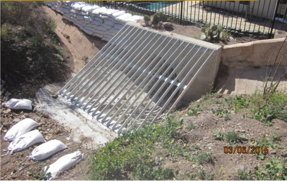
(Trash Rack_Small) (Trash Rack_Small)
